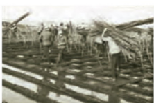
Softwood products workers constructing shield protection for the Afsluitdijk causeway dike (photo W. Verkerk, 1929-1932).
