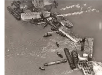
Caissons were also used after the catastrophic North Sea Flood of 1953. Here at Oostwijk (photo K.L.M. Aerecaerts, 1953).
